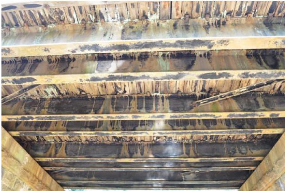
Figure 6 Surface corrosion of main girders of Bridge 62
