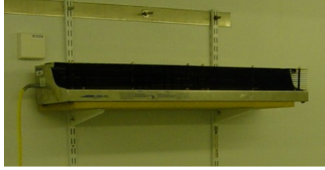
Figure 10: Typical wall mounted upper-room UVGI air disinfection fitting.
