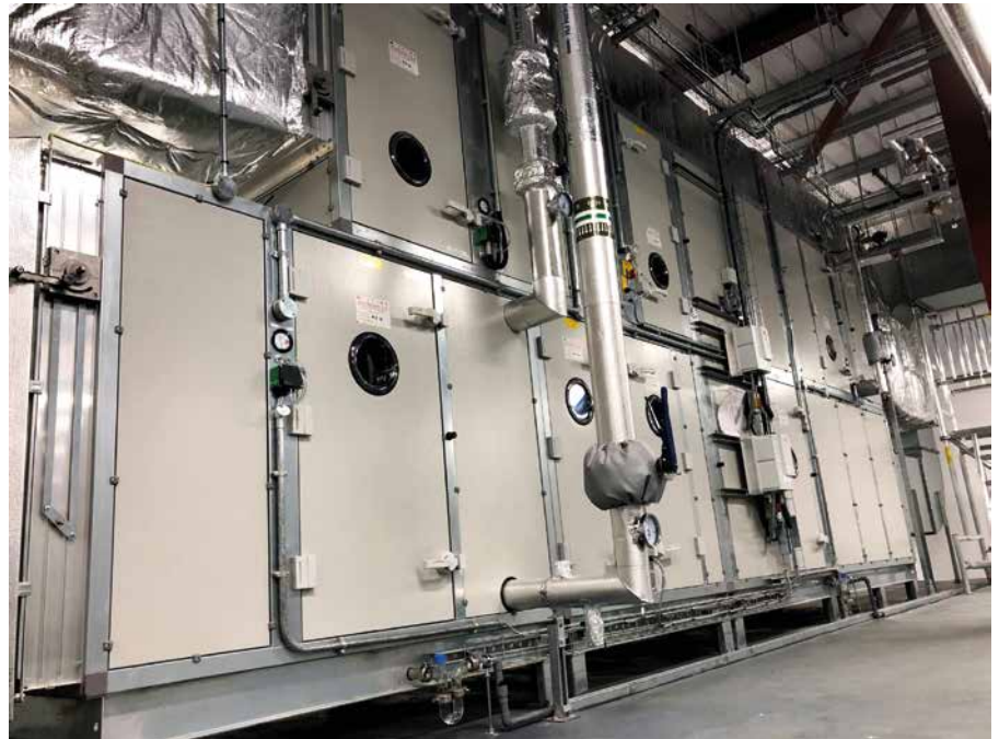
A modern UCV theatre air-handling unit.
